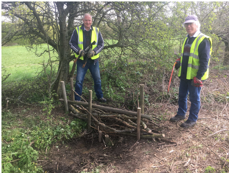
The leaky weir created by John, Colin and Mike
